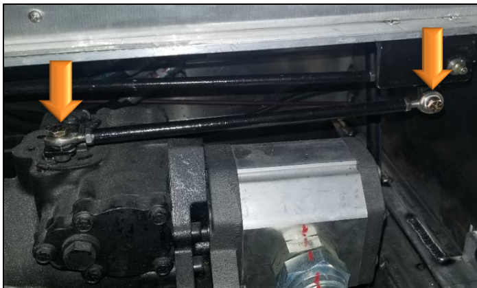
250 HOURS-4: Control Rods
