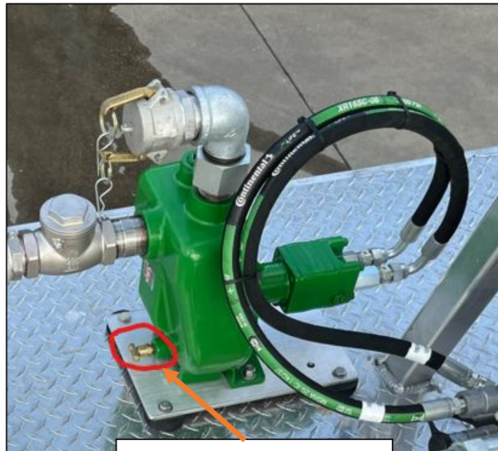
PUMP CASING DRAIN PORT
